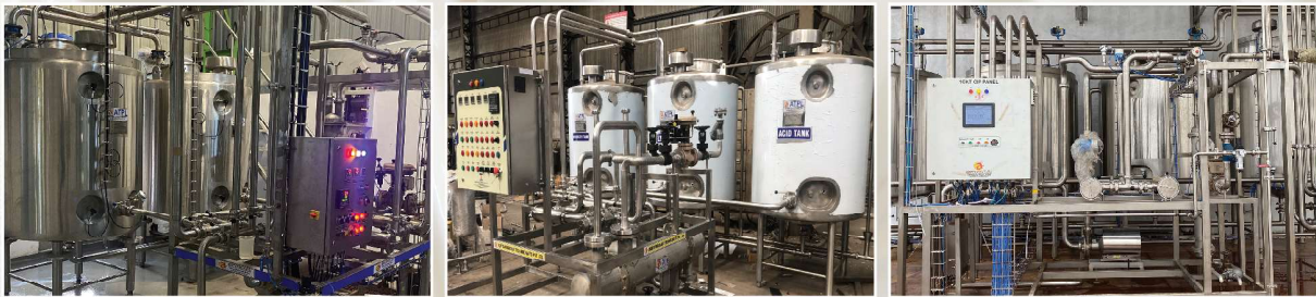
Five Circuit C.I.P. System
