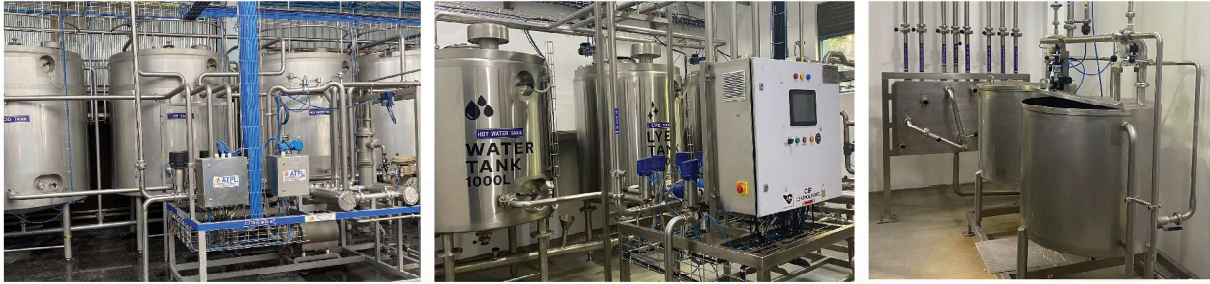
Single Circuit C.I.P. System
