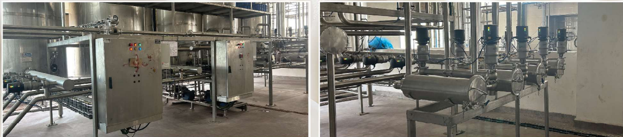
Semi Automatic/Manual C.I.P. System
